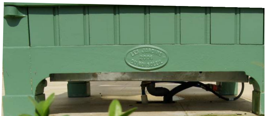
Example of a connection under the planter
